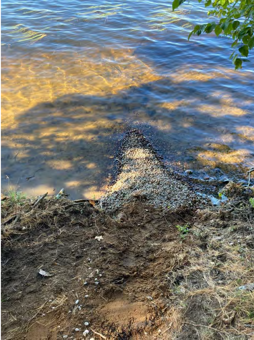
Buried pvc air lines entering lake. The lines were buried at the shoreline interface to hopefully help freezing issues experienced by Halsey Lake.
