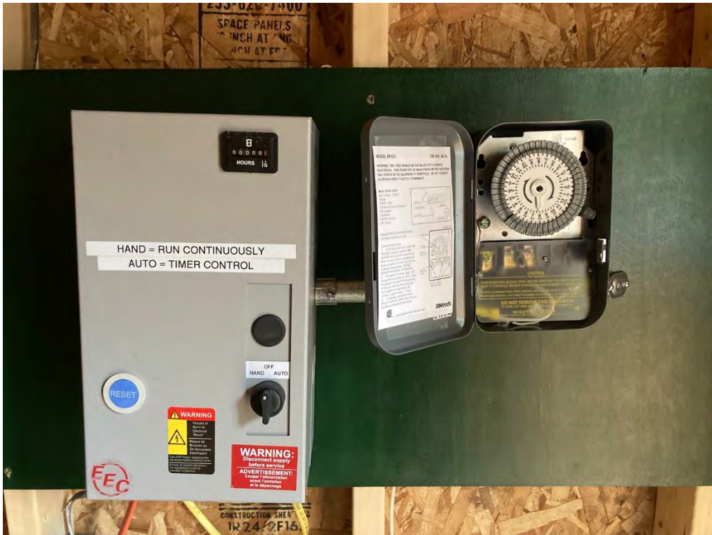
Blower electrical control panel within the pumphouse designed and built by Andy Mott
