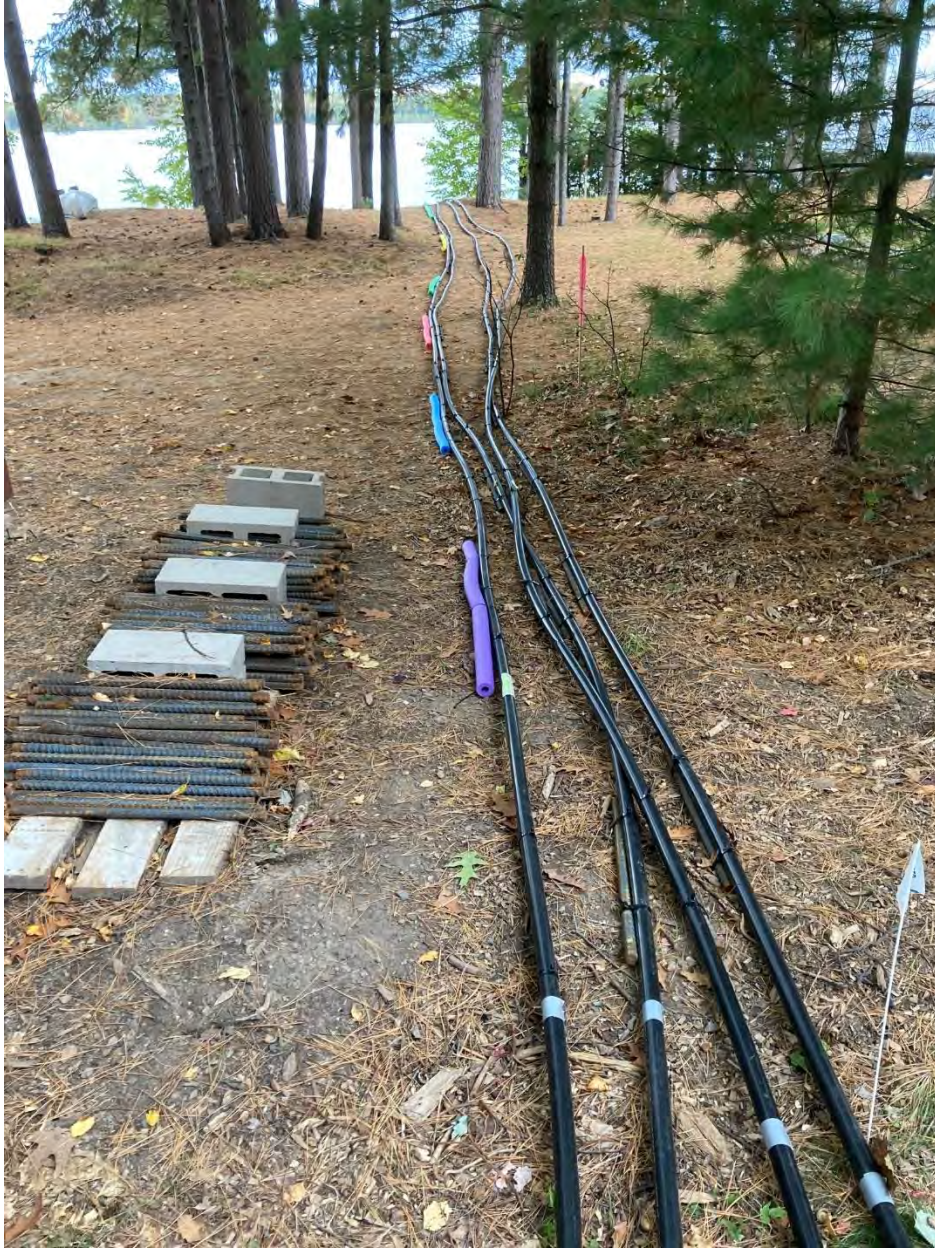
The four pvc air lines laid out to be installed. Note noodles and rebar attached and ready for deployment.
