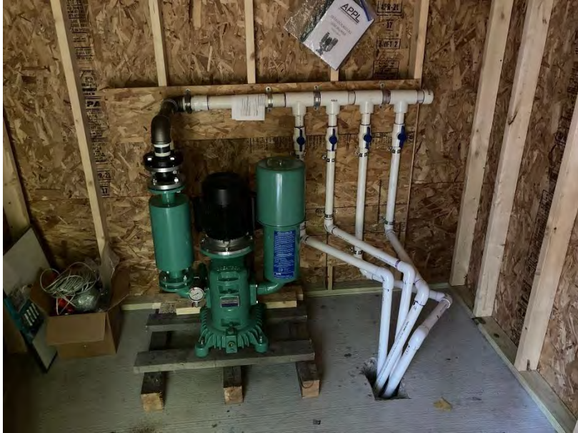
Blower in pumphouse. Note valve system and odd angles of pvc airlines due to undersized 90-degree pvc used to enter the pumphouse.
