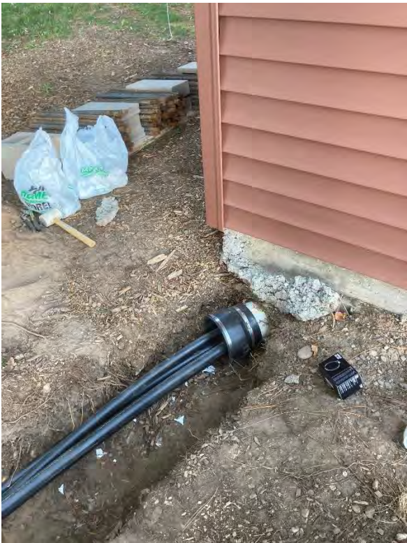
PVC air lines entering Little Rice Lake pumphouse
