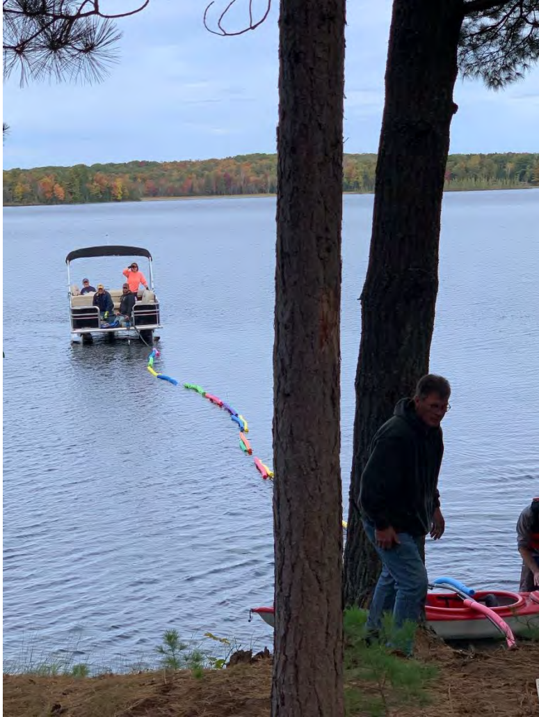
Installing an individual pvc air line in the lake. Note the extra noodles attached to the first 100' and kayak laid perpendicular and ready to be deployed to help with floatation.
