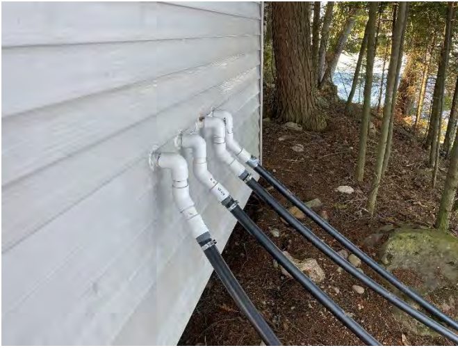
PVC air lines entering Halsey Lake pumphouse for comparison to Little Rice Lake installation.
