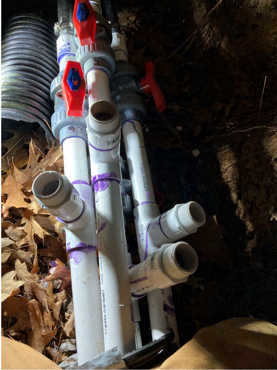
Valve system near lakeshore. Note: valves are shoreward of the T's, and caps are on end of each T in final step.
